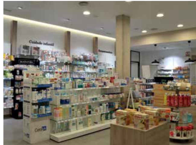
Compatible lighting with installations that require UGR<19
