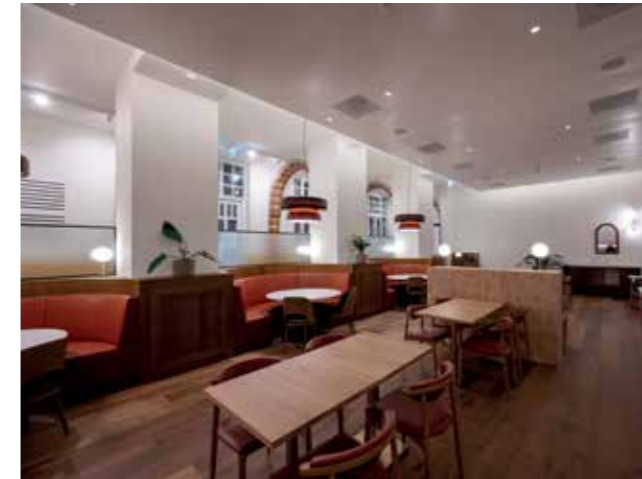
Compatible lighting with installations that require UGR<19
